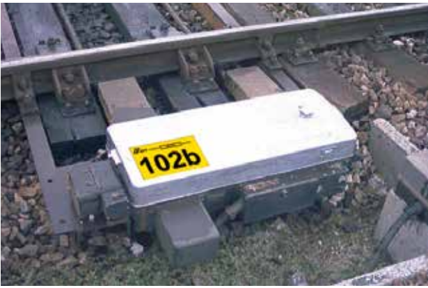
Switch shunting box
